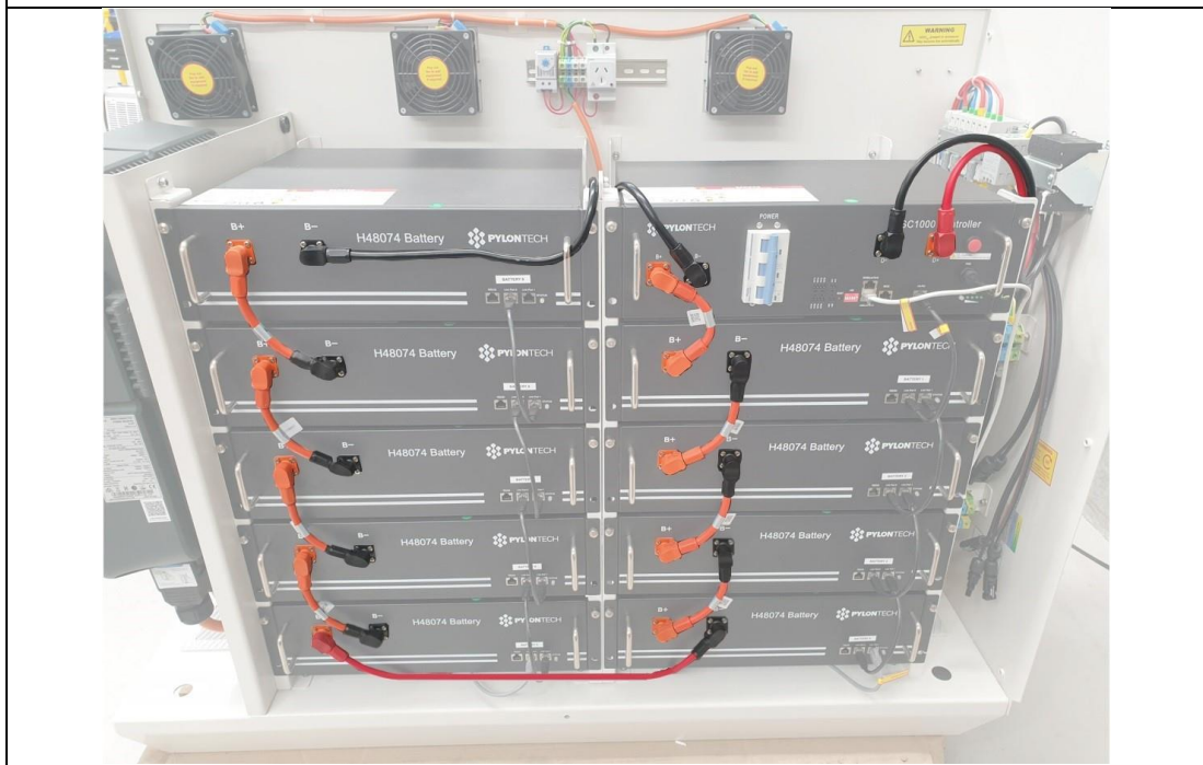
Battery Power Connections
